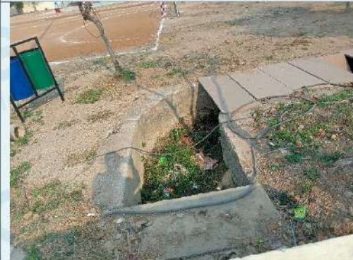
Fig 27: Drainage system for the water movement in the campus
