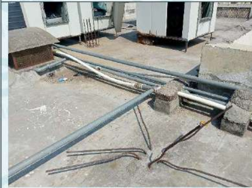
Fig 33 : Pipe supply for water above the hostel
