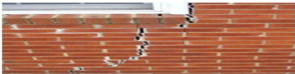
Fig. 1.1 Damage to superstructure of a building
