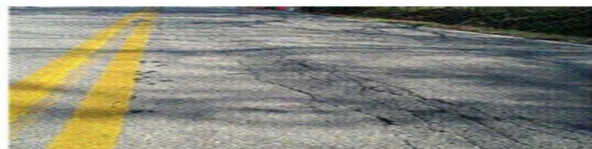
Fig. 1.2 Heaving and cracking of roads
